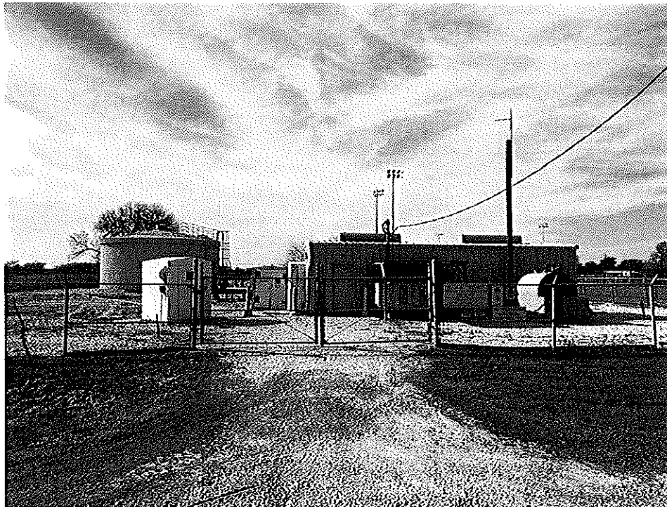
4 - Bishop East PS - this Pump Station is used solely by the Nueces WSC. Originally, the City of Bishop received service from this station as well. The City is now serviced by a city-owned station on the west side of the city.
